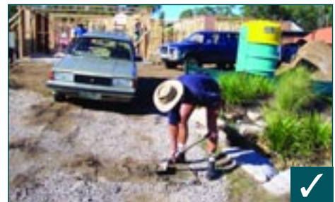
Excessive sediment deposits must be removed from entry/exit point (rumble pad)
