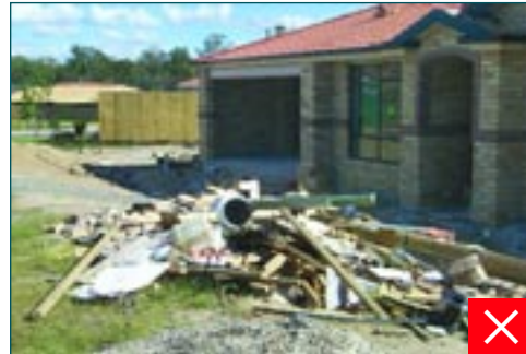
Poor litter and building waste storage
