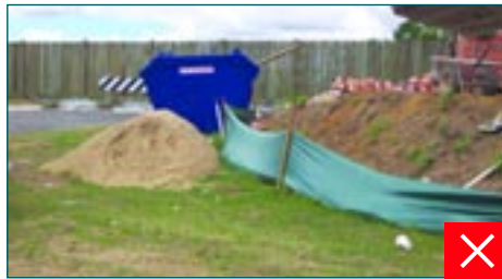
Poor site planning – stockpile outside the sediment fence and building waste not placed in skip
